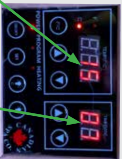
Fig1. POWER & HEATING lights illuminated to show sauna in operation
